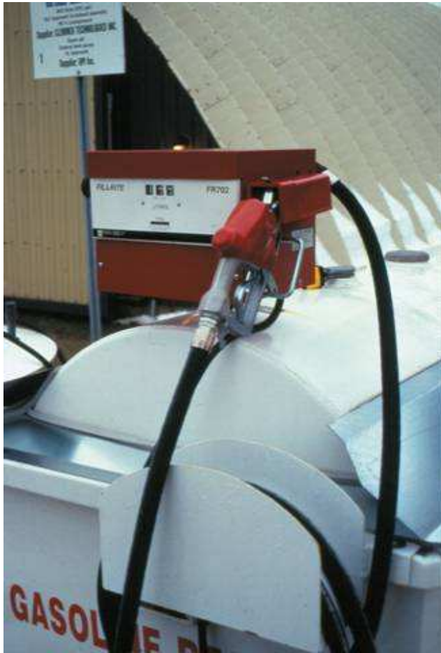
Figure 2. Fuel tanks can be placed in a dike to provide secondary containment in case of a spill.
