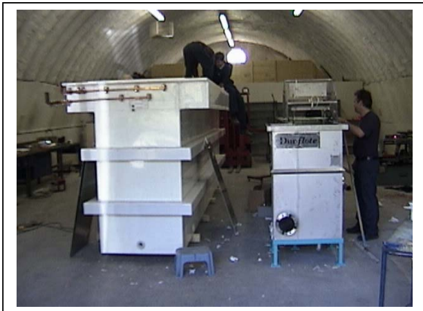
AOP ELECTRO HORIZONTAL AND DAF CLARIFIER
